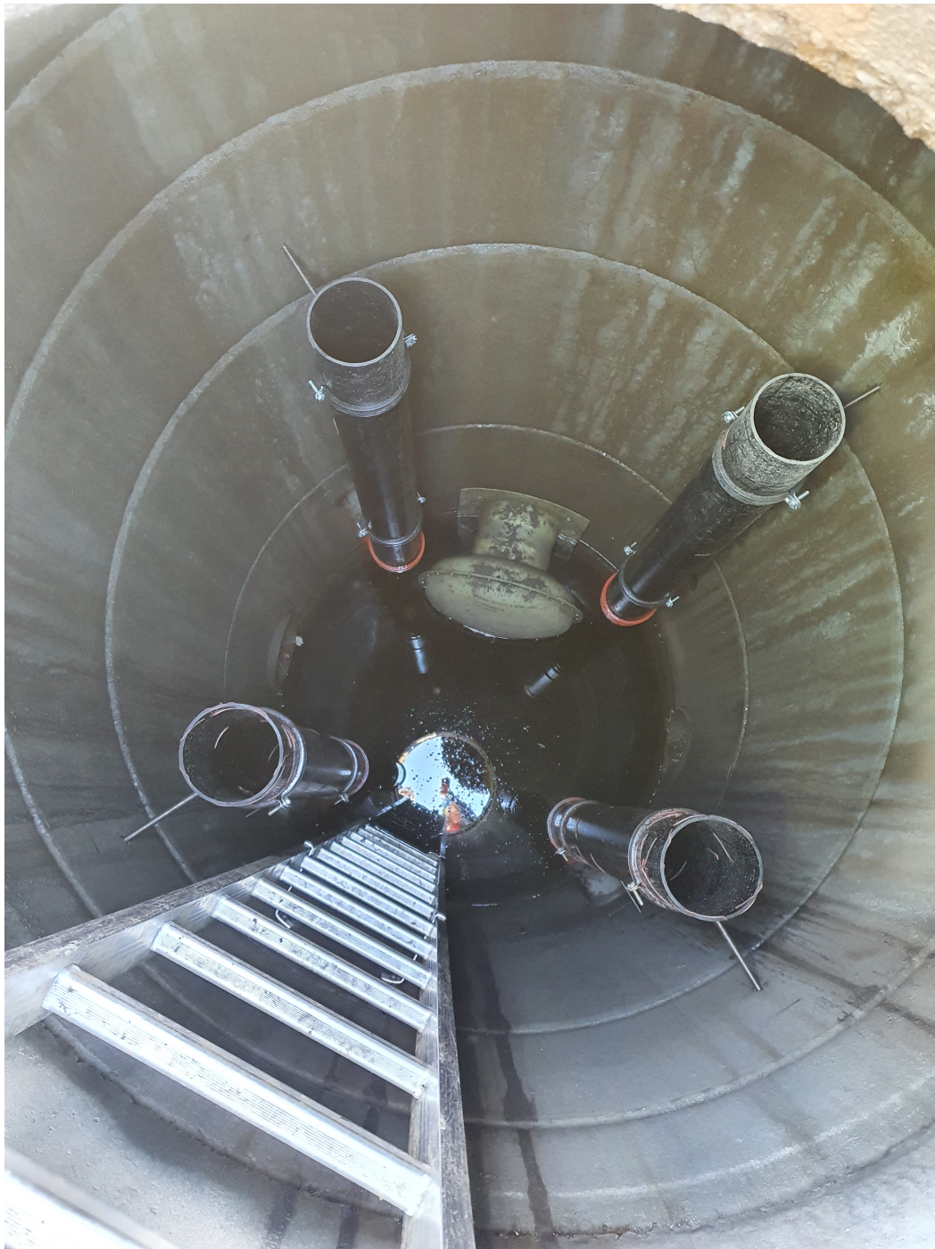
Figure A3.2: The manhole downstream the detention basins in the field pilot. The four vertical pipes are connected to the infiltration pipes as an outlet if the detention basins go full, and the swirl chamber regulates the outflow from the detention basins. Photo credits: Ida Hovland Haveraaen
