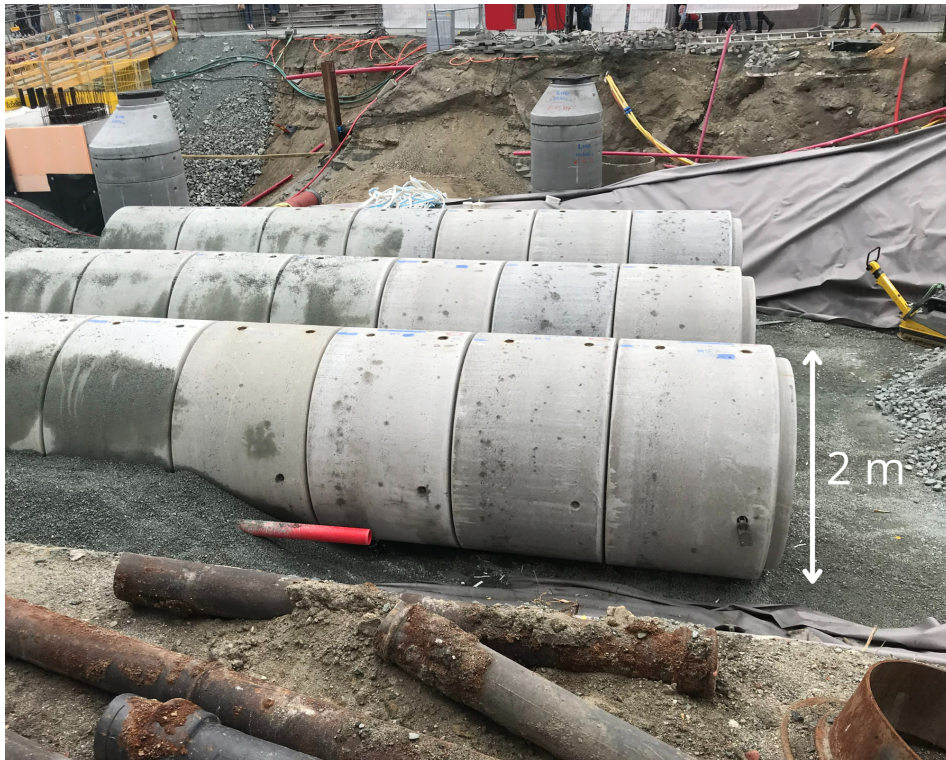
Figure A3.3: From the construction site of the field pilot. The red pipe is the infiltration pipe. The three concrete constructions are the detention basins. Credits: Edvard Siversten (SINTEF)
