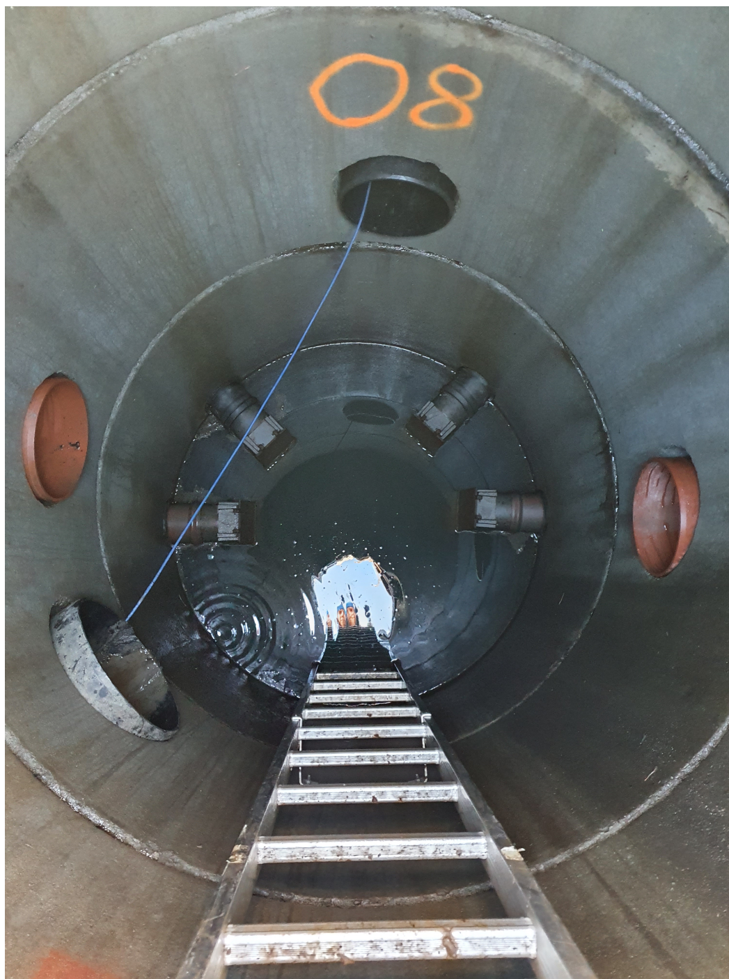
Figure A3.1: Inside manhole O8 in the field pilot. The infiltration pipes are in the bottom, the pipe south-west is the outlet pipe from the catchment area, and the last three are inlet pipes to the detention basins. Photo credits: Ida Hovland Haveraaen
