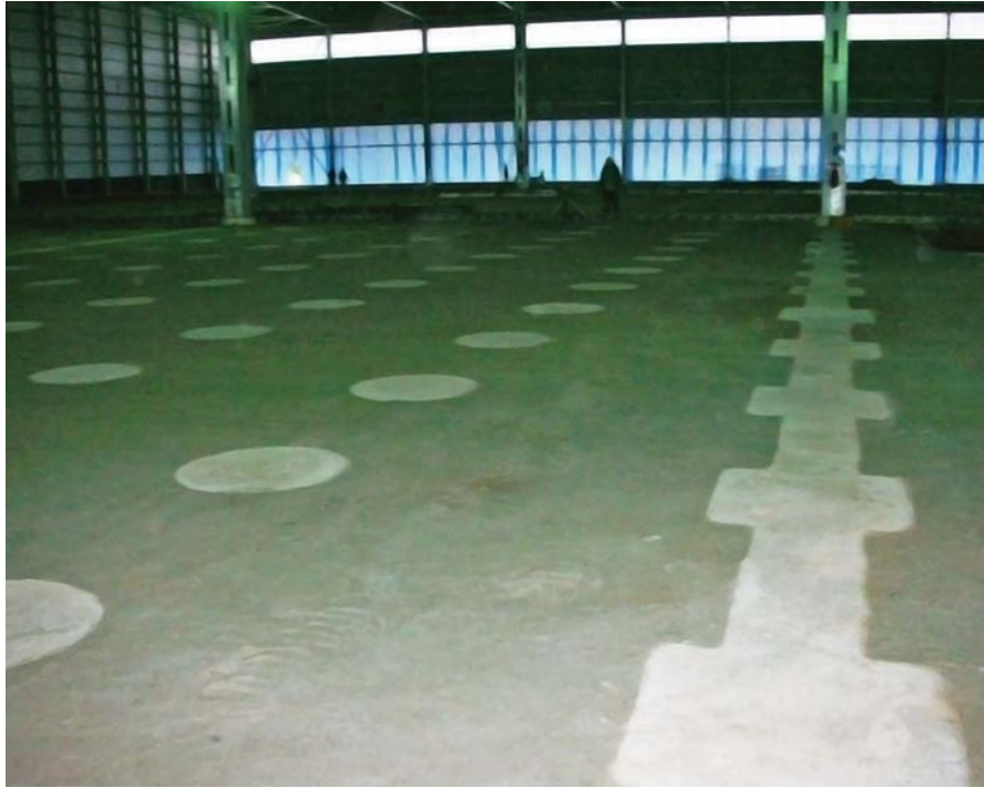
Figure 2: Layout of pile heads and sub-base underneath a pile supported slab (Hulett, 2011).
