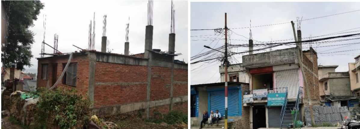
Figure 5-13 Pictures of buildings with typical design, concrete and masonry bricks. The columns with protruding rebar make the building ready for extension at a later occasion.
