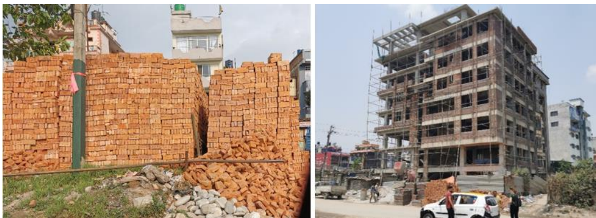
Figure 5-4 Masonry used in the inner walls to the left. The picture to the right show a finished facade with red bricks.
