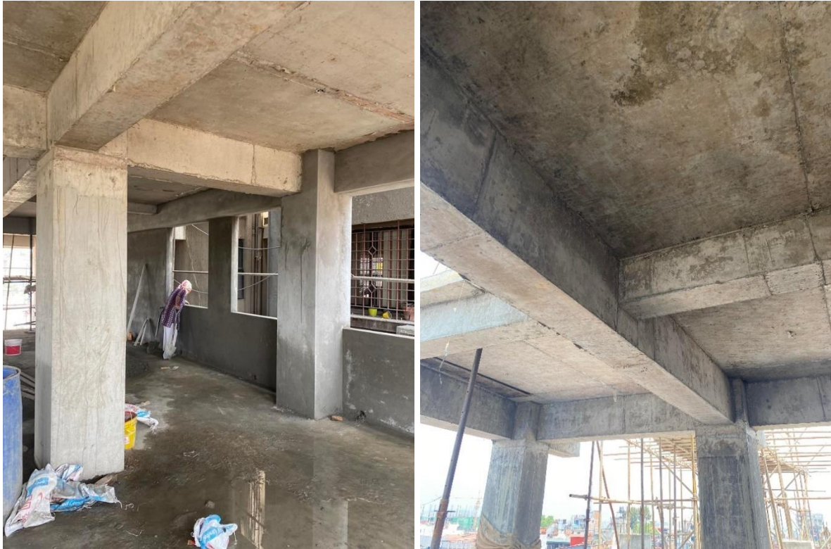
Figure 5-2 The left pictures shows a connection between the column and beams. The right pictures show a secondary beam meeting one of the main beams.
