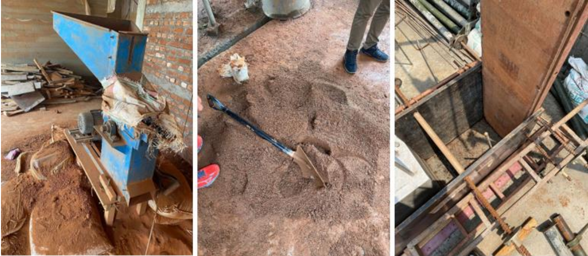
Figure 5-7 Construction of rammed earth walls. To the left, the machine is used to crush the clay. In the middle, a mixture of clay, sand, gravel, and cement are worked up. To the right, a framework is presented.
