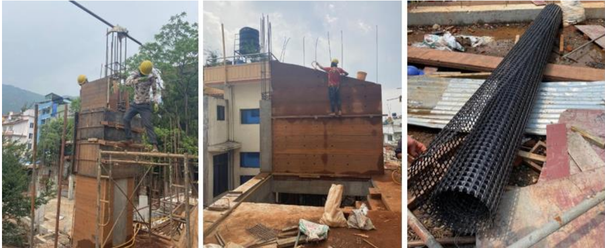
Figure 5-8 Picture to the left shows two construction workers removing the framework. The middle picture shows a construction worker filling the holes with earth. In the picture to the right the plastic used as reinforcement, is shown.
