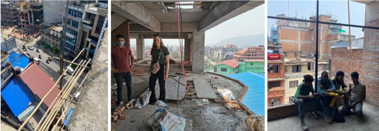
Figure 5-12 Pictures from some of the construction sites. To the left is a scaffold built with bamboo. The middle and right picture is taken at one of the higher floors. The shafts and end of the slabs are not secured. The workers sit unsecured at 5 th floor. As the pictures illustrate the HSE should be improved.
