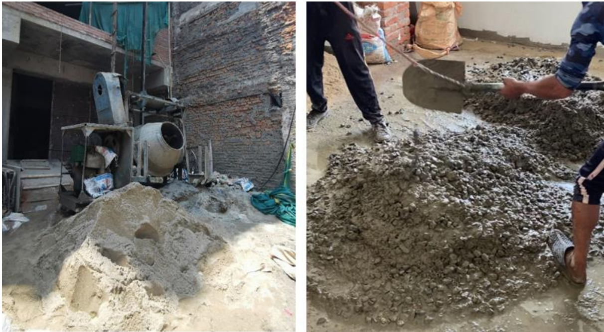
Figure 5-3 Alternatives for mixing of concrete at the construction site. To the left is the mixer shown. Right picture illustrate how they sometimes mix the concrete
