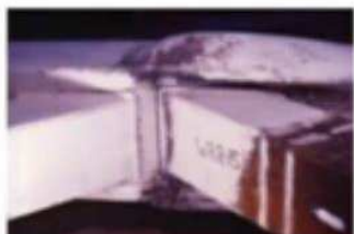
Chord side wall buckling
