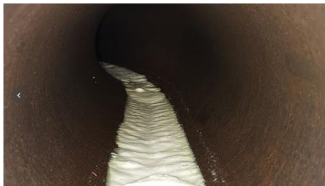
Figure 25 Inside 5D bend. Corroded surface from fabrication and initial testing with water
