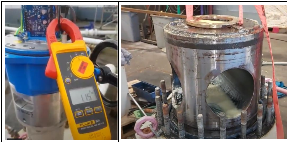
Figure 21 Metering of current during actuation. Internal hub in FDV lifted out for inspection. Notice glider rings (black) at top. Samples from oil/wax slurry was taken for later analyse.
