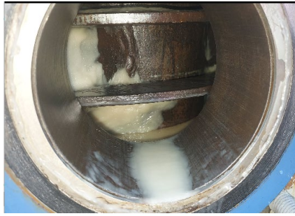
Figure 14 Inlet port Pig Diverter. Notice blocking bars (2 of) that prevent pig from entering in to void. Similar will be fitted on outlet port
