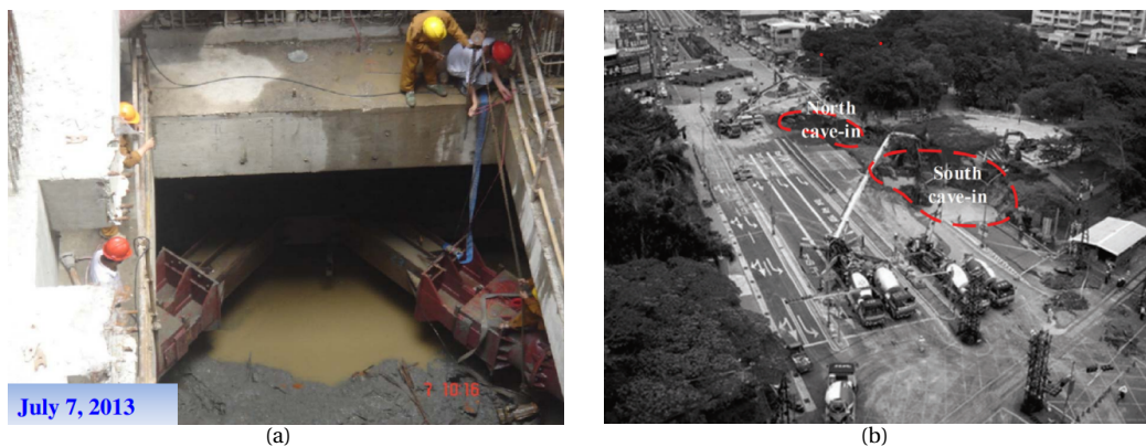
Figure 2.1: In-situ photos for excavation leakage accidents: (a) pit corner in the northwest on July 7, 2013 in a subway station in Shanghai ( Tan and Lu, 2017 ); (b) north and south cave-ins in tunnels LUO09 in Kaohsiung ( Cheng et al., 2019 )
