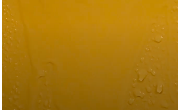
Figure 4.7: Water film on exterior side of panel. Photo taken during test no. 195 with HPL panels and a sealed top joint.
