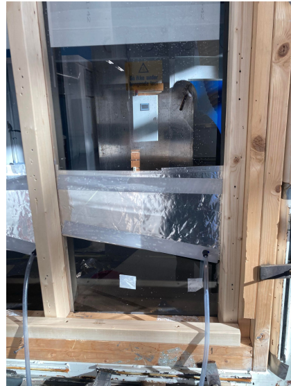
Figure C2: Tape placement for gutter system on Lexan board. Double-sided tape is used.
