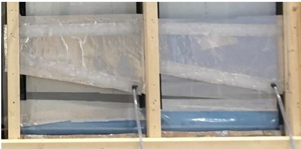
Figure 4.30: Gutter system seen from the interior side. Aluminium gutters above the blue plastic gutters.
