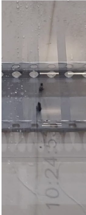
Figure 4.17: Crack in Fiber Cement White caused by extra fastening points, seen from the interior. Caused before testing with "U + FP" in test no. 118.
