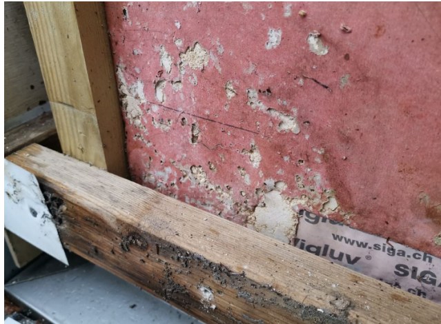
Figure 1.1: Large amounts of water intrusion through both vertical and horizontal joints in an apartment block in Bergen. One consequence is a decomposing wind barrier (Geving, 2022).
