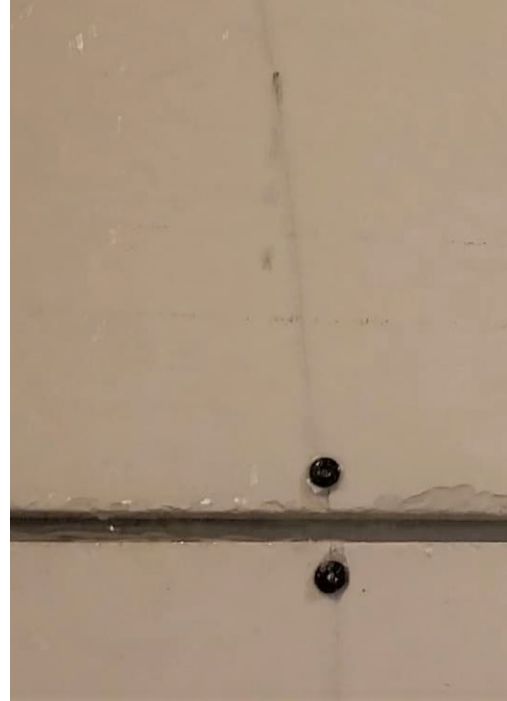
Figure 4.18: Crack in Fiber Cement White caused by extra fastening points, seen from the exterior. Caused before testing with "U + FP" test no. 118.
