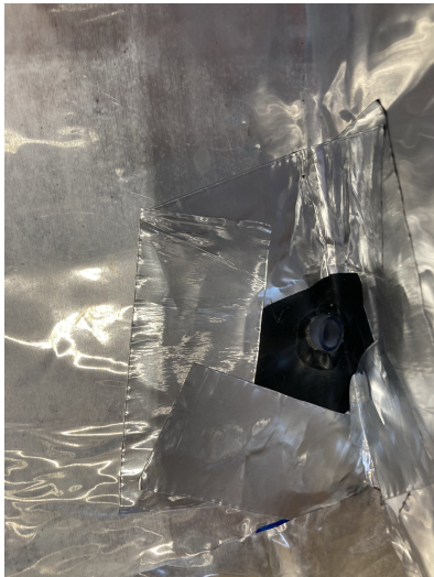
Figure C3: Closeup of a sleeve placed at the bottom of the gutter with a tube pulled through. The perimeter of the sleeve is sealed with aluminium tape.
