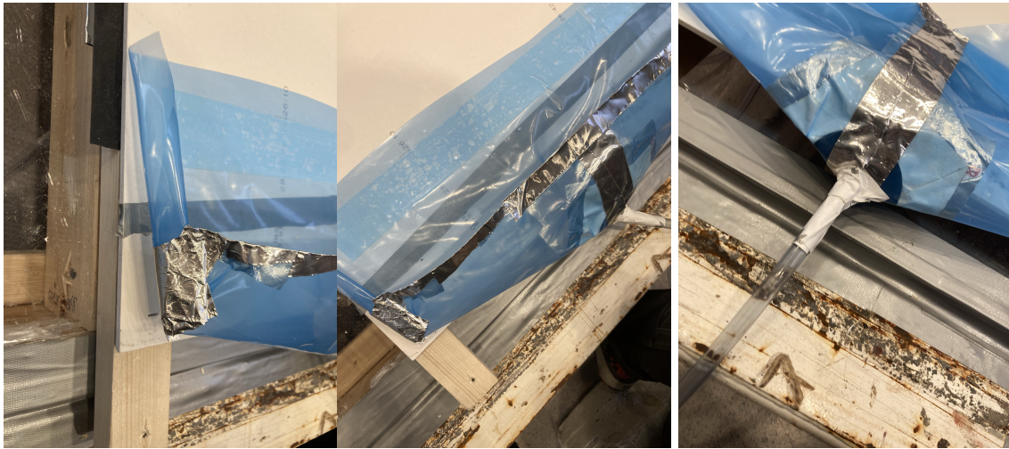
Figure C12: The foils were then cut and trimmed to a fitting shape. The sides of the gutter was ensured watertight by folding them behind and taping with aluminium tape
