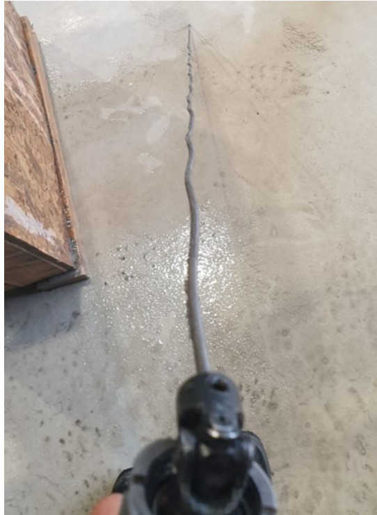
Figure 15.12: Rod twist off during drilling.
