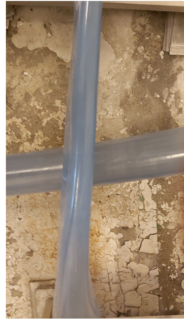
Figure 4.1: An image of the constrained tube, with an unconstrained tube behind. Both these tubes are rated for atmospheric pressure, and the constrained tube is the one connecting the primary tank with the primary pump. This tube experienced constraint with the use of the higher settings of the primary pump.
