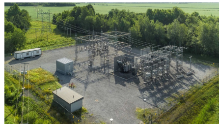
(b) A digital substation
