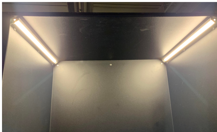
Figure 26: New lighting in the control room.
