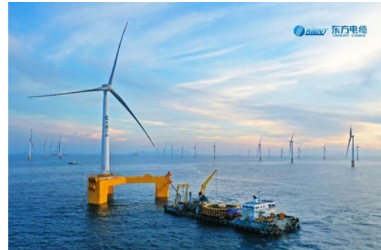
Figure 5.12: A cable laying vessel performing dynamic cable assembly at China's Yangxi Shapa III pilot project [78]
