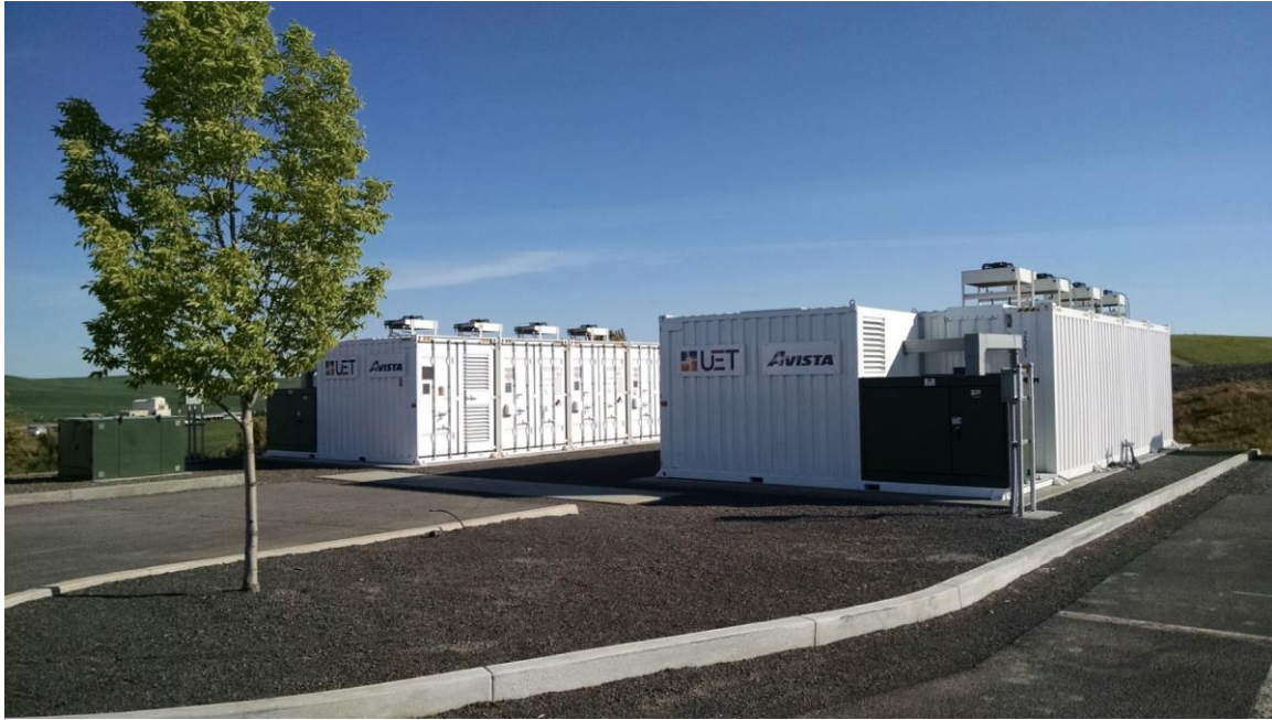
Figure 2.17: 1 MW 4 MWh Containerized vanadium flow battery. Source: Wikimedia Commons [26]
