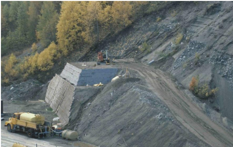
Figure 3.1: Picture of the finished slope with the permanent berm on top (Fannin and Hermann, 1990)
