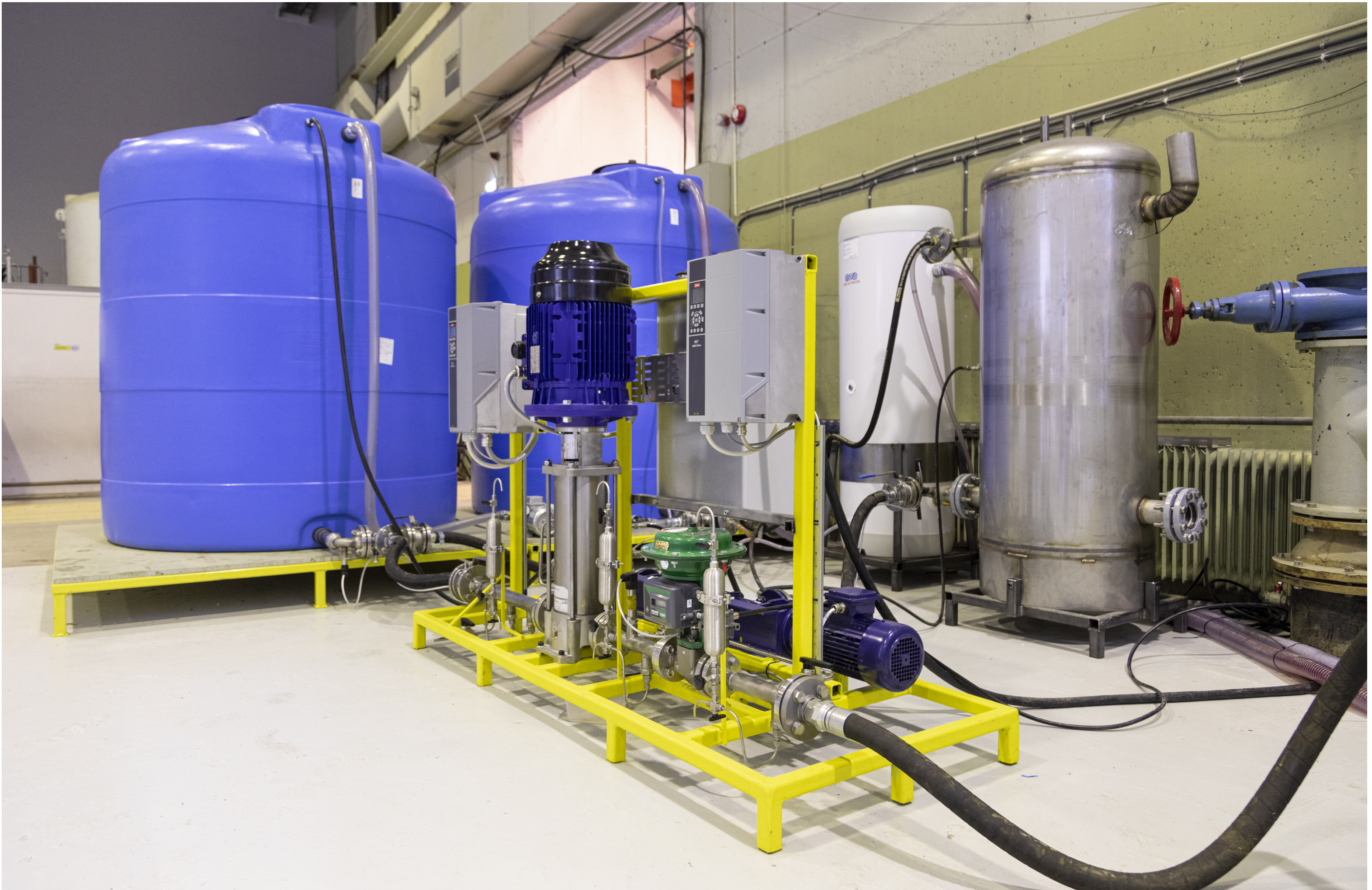
Figure A.5: A picture of the pump system installed at the test-rig.
