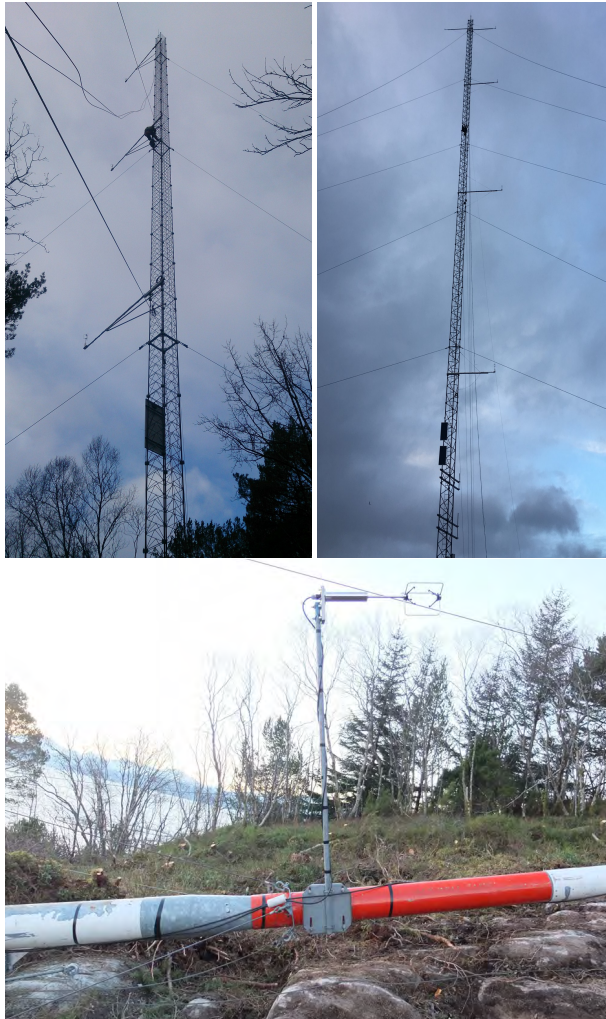
Figure 4: Examples of mast structures used. Rectangular lattice tower at Aakvik in Halsafjorden (upper left), Kvitneset in Sulafjorden (upper right), and Halsaneset in Halsafjorden (below), where one of the anemometer can also be seen. Photos: Kjeller Vindteknikk.
