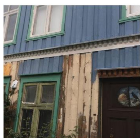
Figure 5. Deteriorating façade (NTNU).
