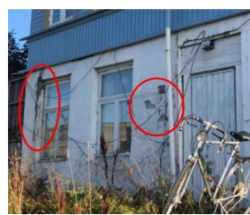
Figure 11. Humidity damage (NTNU).
