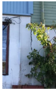
Figure 10. Crack between the buildings Strandveien 19 and 21 (NTNU).
