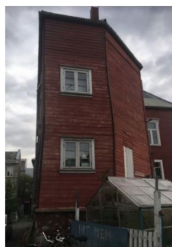
Figure 6. Leaning house (NTNU).
