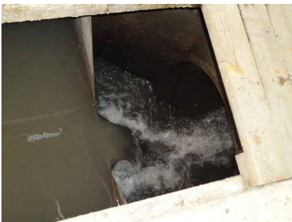
Figure 76: The V – notch weir
