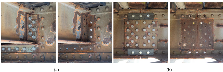
Figure 4.4: The damage types imposed on the bridge before and after damage. (a) Damage type 1. (b) Damage type 4.
