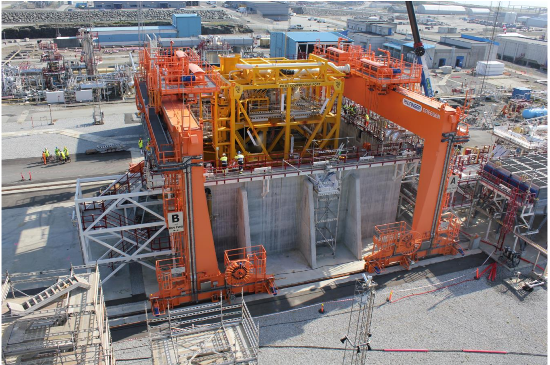
Figure 3 Åsgard subsea compressor pilot module lifted into test pit at K-Lab
