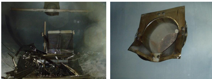
Figure 6-2: Damage to Field-B GOSP Low Pressure Separator
