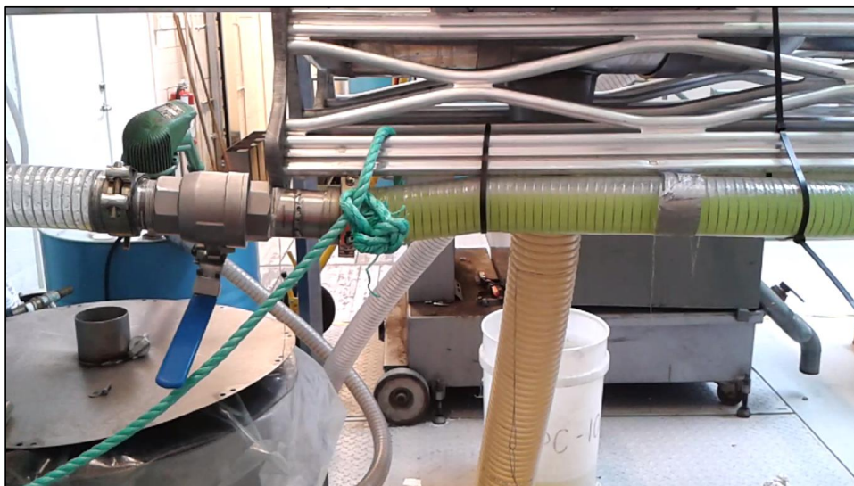
Figure 10-12: Accumulation of Liquid at the tight Valve Opening
