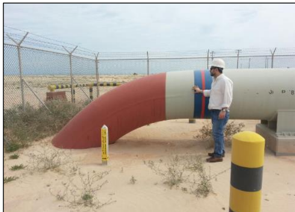
Figure 7-1: TL-10 Pipeline (42 inch)
