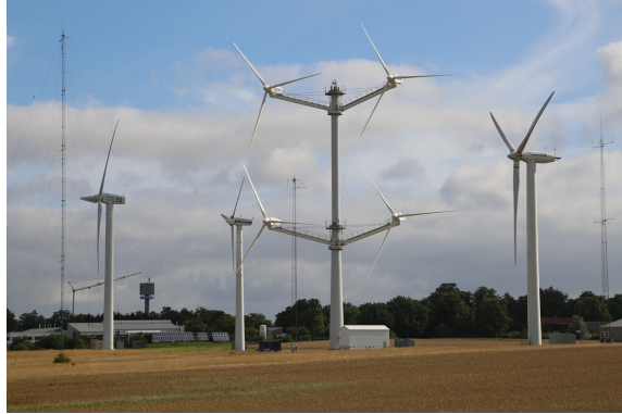
(b) The MRS prototype by Vestas installed at Riso [24]
