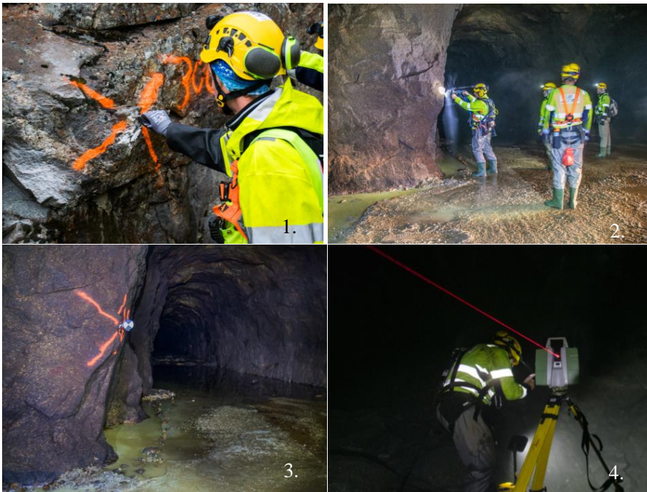
Figure 3. 3D scanning step-by-step process and resulted scan (1 - bolt location marking; 2 - drill for bolt placement; 3 - scanning target placement; 4 - laser scanning)
