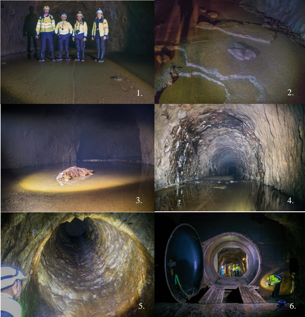
Figure 2. Field visit during dewatering of Roskrepp headrace tunnel (1 - asphalt lining; 2 - scalped asphalt section; 3 - rock fall; 4 - possible weakness zone; 5 - UST shaft (see figure 1); 5 - adit plug before penstock (see figure 1))
