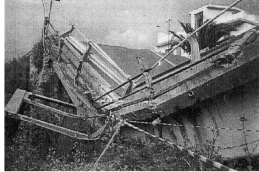
(b) The collapsed St.Stefano bridge [13].
