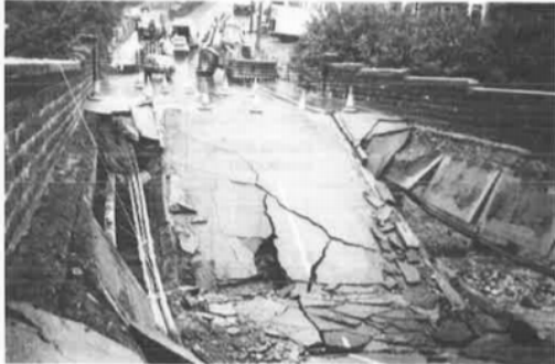
(a) The collapsed Ynys-y-Gwas bridge [4].
