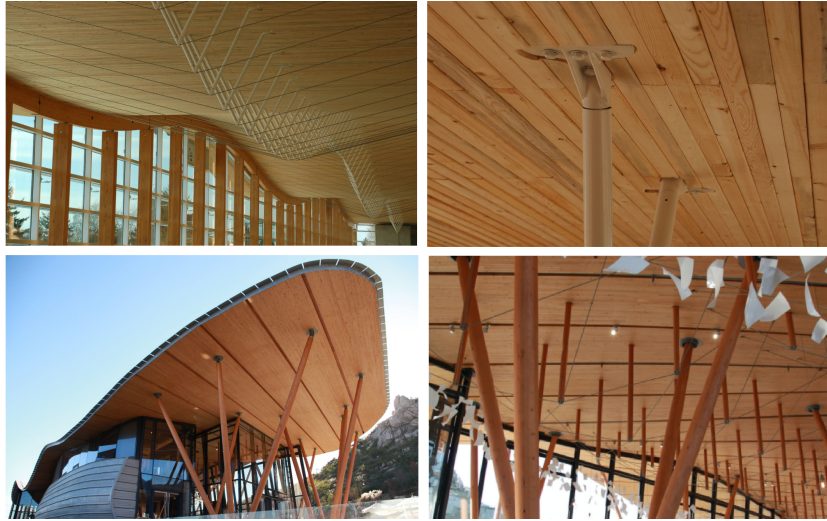
Figure 2.12: NLT roof structures by StructureCraft. From upper left: (1) and (2) Samuel Brighthouse School Atrium, (3) and (4) Tsingtao Pearl Visitor Centre. From Structure-Craft’s website
