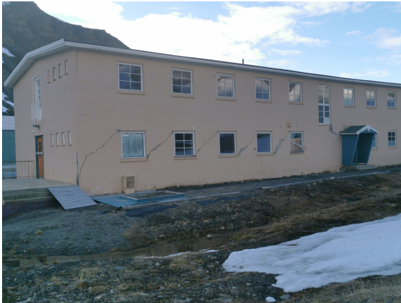
(a) Abandoned building in Longyearbyen, which had to be evacuated after a power failure in the cooling system. Cracks in the walls of the house are visible (Photo taken by the author).
