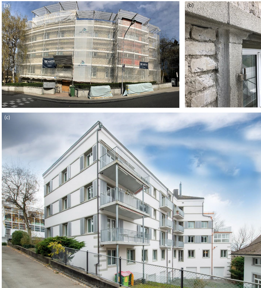
Fig. 13. Multi-family home in Zurich, Switzerland: (a), (b) during and (c) after the retrofit in 2020 with silica aerogel blankets. The existing render was removed (see detail in (b)), 20 mm of silica aerogel blanket were applied and covered with render again, resulting in the final state as shown in (c) (opposite view of the building). Neither the roof nor the characteristic stone details on the building façade and around the windows had to be modified. Images: AGITEC AG.
