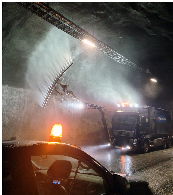
Figure 2: Tanker with nozzle equipment, washing shotcrete tunnel lining of the Grillstad tunnel in Trondheim, Norway (Photo by T. Meyn, 26.03.21).
