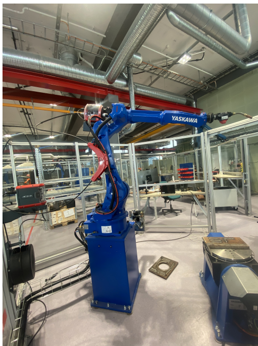
Figure 4.1.: Yaskawa Motoman GP25-12 with welding equipment as installed at Perleporten
