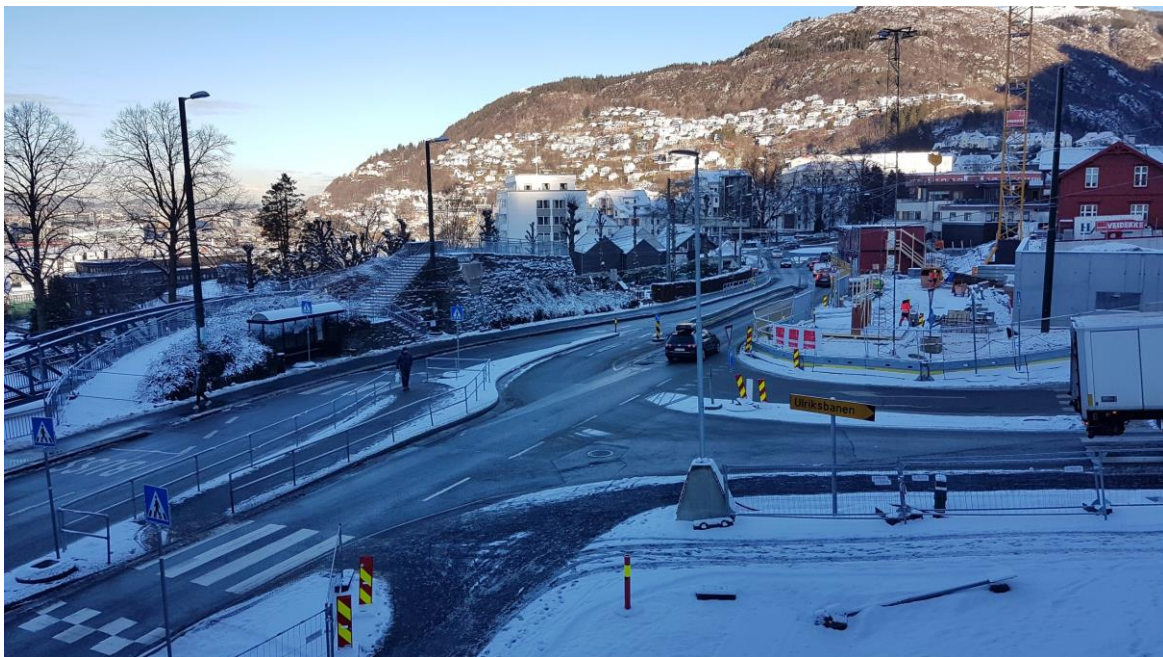
Figure 3.12: Construction work on the northern side of the tunnel north of intersection 2
