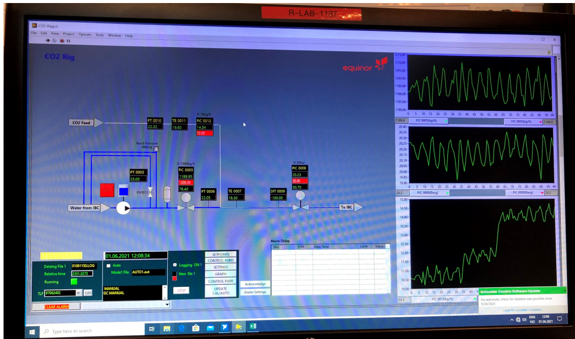
Figure 12: Controlling and monitoring screen of CW rig
