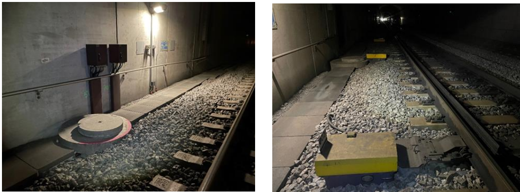
Figure 2 Cables casing (left) connected to the switch (right)
