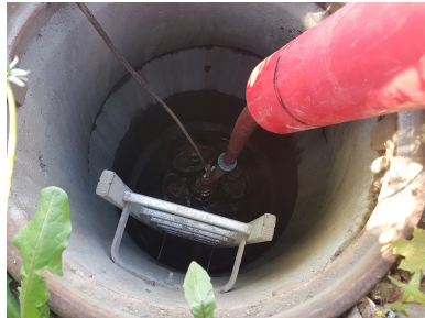
(a) Hose connection to the water distribution network
