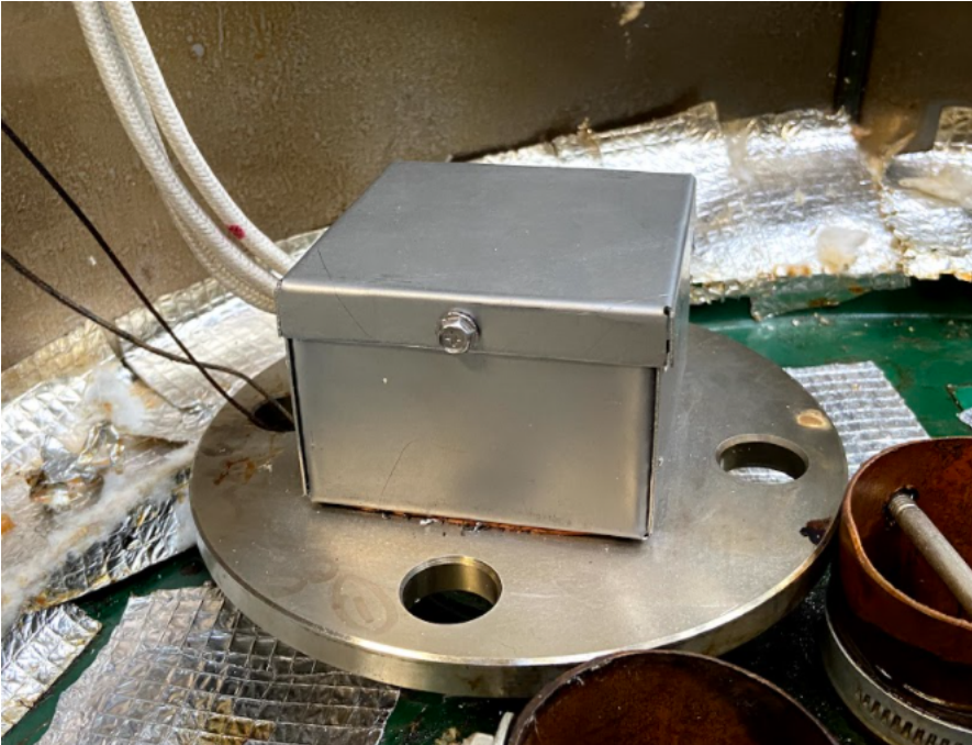
Figure 16: The new metal housing for the heating element
