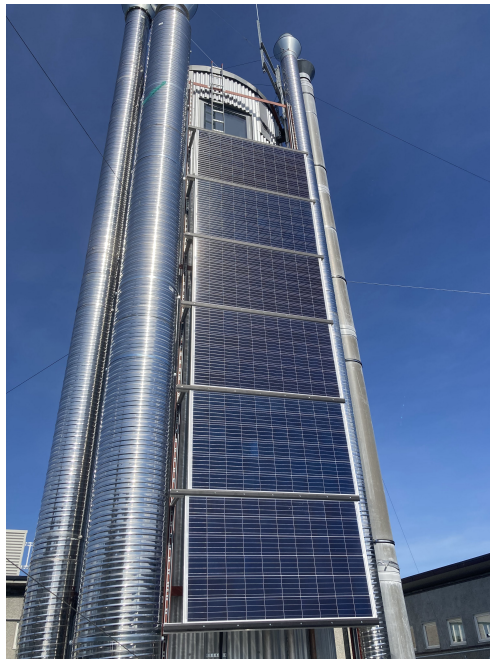
Figure 9.1: The PV panels used.
