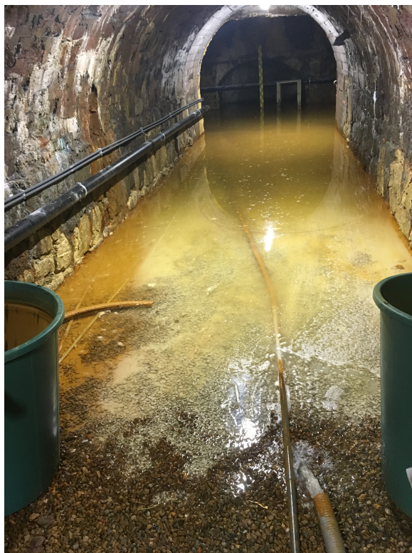
Figure 2.11: A picture taken of the water in the Killingdal tunnel, that can be described as acid mine drainage (AMD) water.
