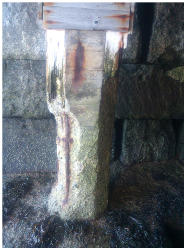
Fig. 2.2.2. Exposed corroded steel reinforcement. Image was taken on Pier 2 in Narvik, 2018.
