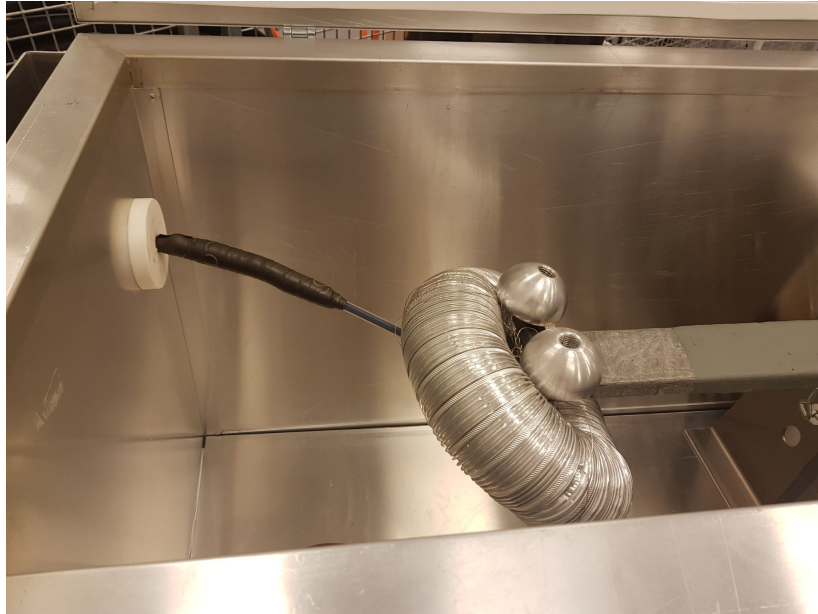
Figure 12: Connection to the conductor of the bar. Some corona protection is added for the other project.
