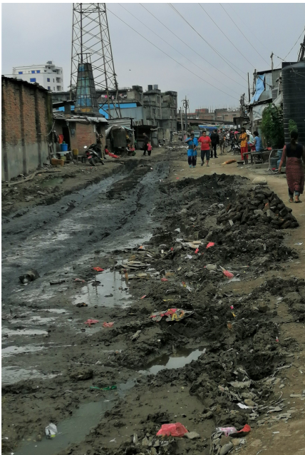
(a) Street of Balkhu slum. The picture displays the condition of under construction street due to leakage of sewage pipe.
