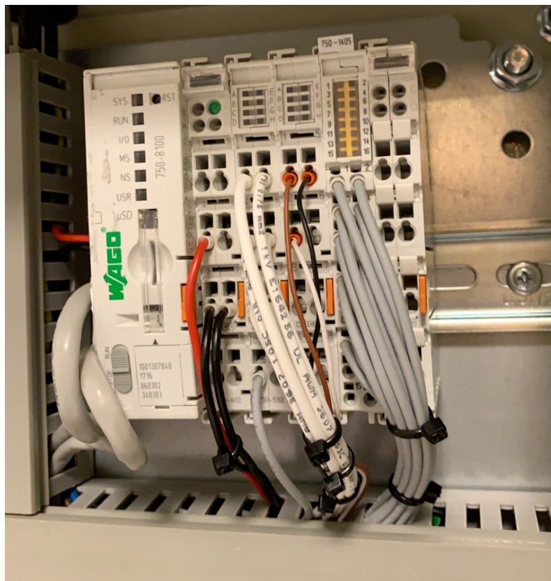
Figure 61: PLC with I/O modules
