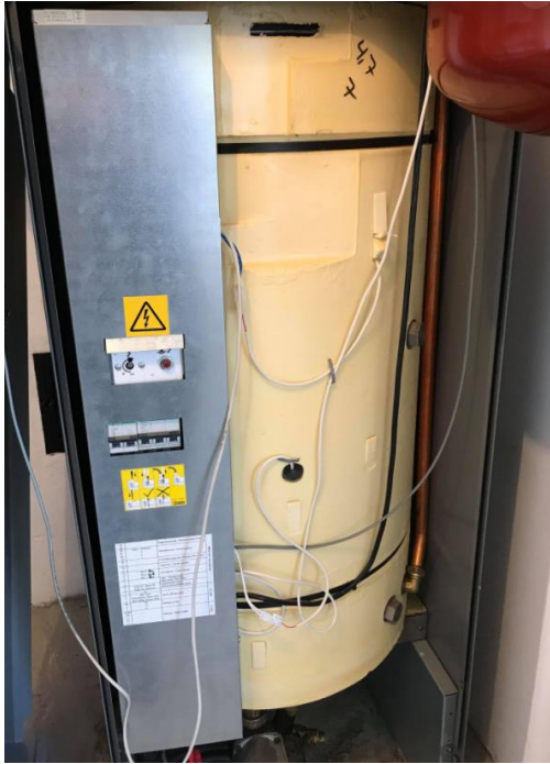
Figur 11, Installert EcoEl framsiden
