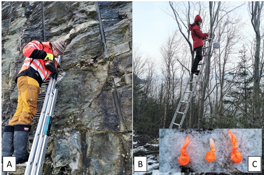
Figure 3.2: A) Installation of rock temperature loggers using a drill and silicone for sealing. B) Installation of radiation shield for air temperature loggers. The second box was installed in a lamp post. C) Photo of three loggers, encapsulated in rubber pockets and colored visible.
