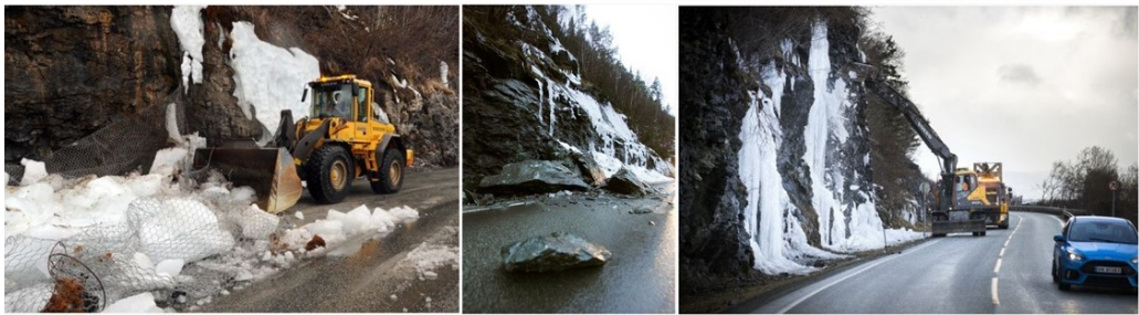
Figure 1.9: Photos from Bynesveien captured during previous years, showing removal of ice along the road, and one of many rock falls reaching the road. The figure to the right is taken on the 21st of March 2019. The date is unknown for the two other photos. Photos: Agnethe Weisser, Rune Petter Ness, Morten Antonsen (Adresseavisen, 2020).
