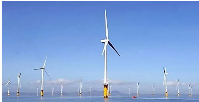
Figure 1. 1: Offshore Wind Turbine Farm [4]
