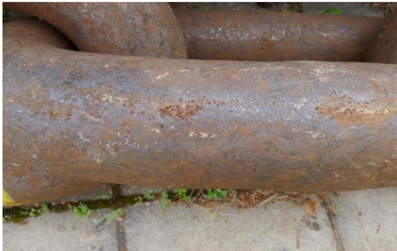
Figure 20: Typical corrosion found in zone 2. Picture of chain used at Åsgard A [14]
