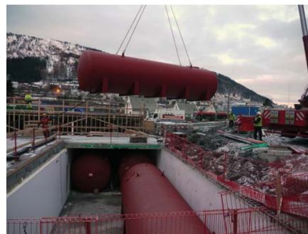
Figure 58: Flat-ICE container HVL Bergem [72]
