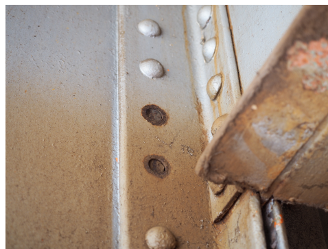
Figure 1.1: Damaged joint (Photo: Gunnstein T. Frøseth).
