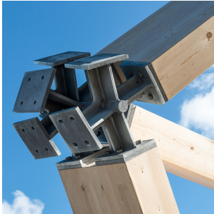
(a) Connector detail at the Crossrail Place in London. The connectors consists of welded steel plates connected to the timber by glued threaded rods. Photo: ©Nigel Young (Seele, 2014).
