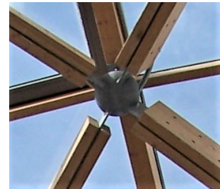
(c) Connector Detail at The Herbert Art Gallery & Museum in Coventry, England. The splices are welded to a sphere in the centre. Photo: Cmglee (2011)
