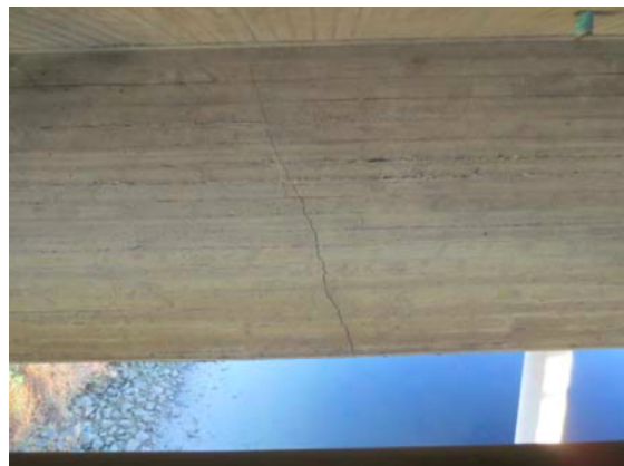
Figure 4.11: Severe cracks found in zero moment section north of axis 8 [32]
