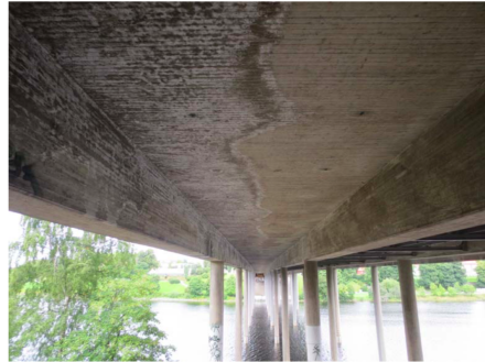
Figure 4.8: Observation of water exposure on outer beam [32]
