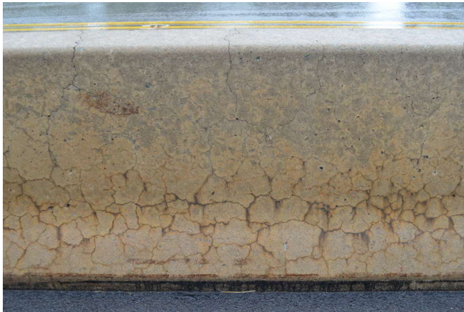
Figure 2.3: Characteristic map-cracking in concrete due to ASR [7]
