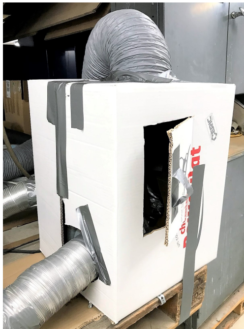
Figure 5.4: Cardboard box installed at the exhaust air outlet in order to fit the VOC sensor.
