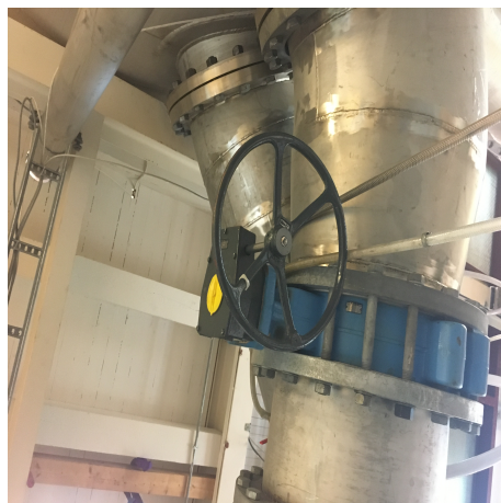
Figure D.4: Manual valve on lower part of the pressure tank
