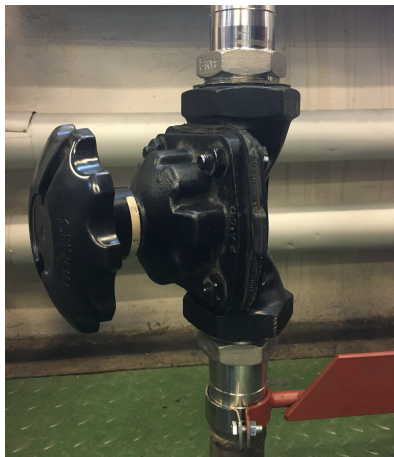
(b) Manual valve at the outlet pipe.
