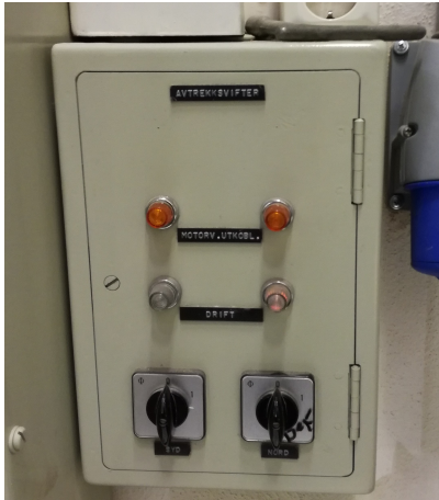
(a) Ventilation fan.
