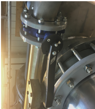
(a) Manual valve on inlet pipe.
